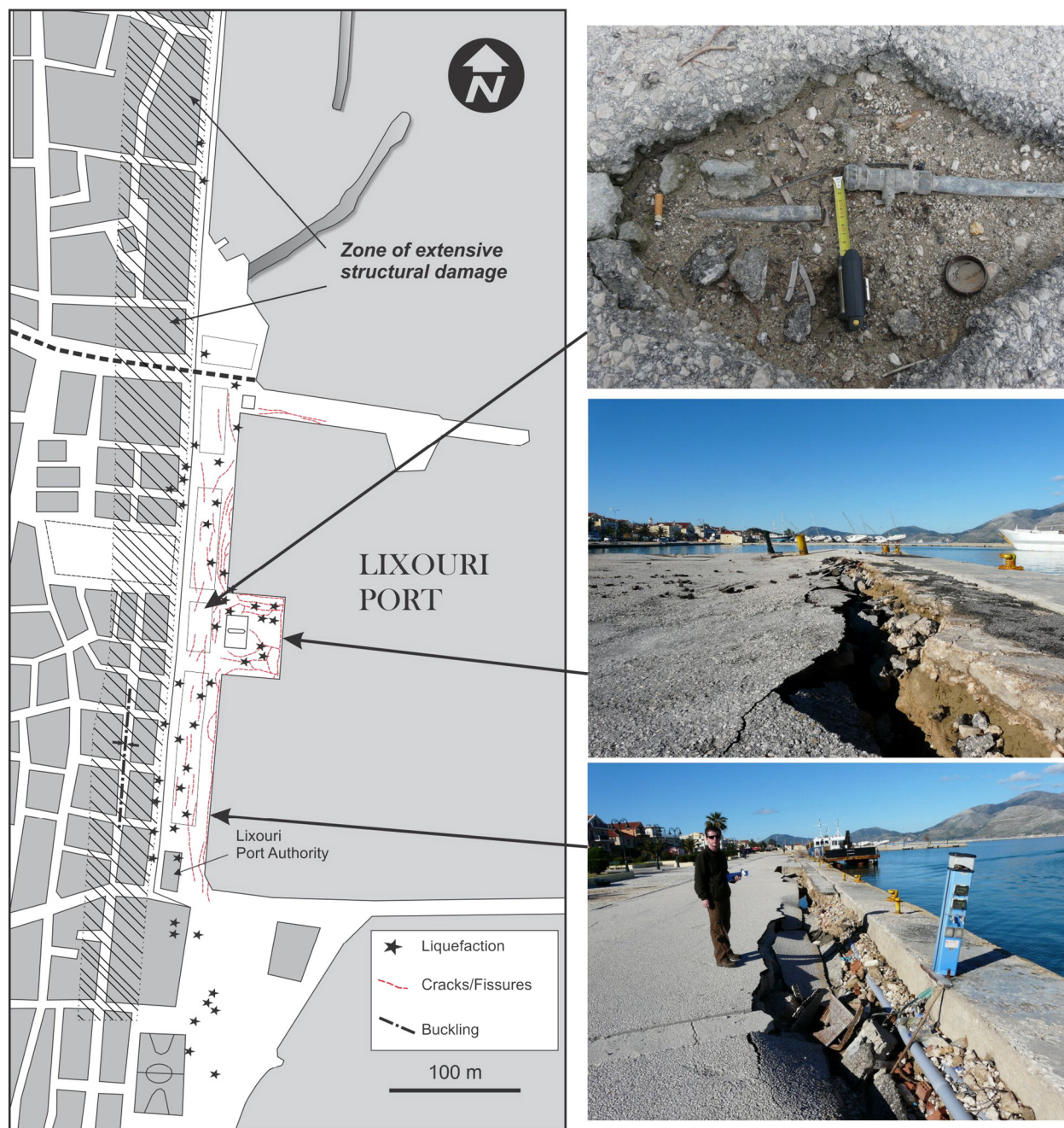
Fig. 7. Map showing the liquefaction manifestation (black star), the cracks/fissures along the waterfront area and the location of buckling phenomena in the town of Lixouri. In addition, characteristic liquefaction-induced structural damages are shown in post-Feb 3, 2014 field photographs (photos taken on Feb. 7, 2014) on the right and particularly a broken water pipeline due to the sloshing of the ground (top), a “graben” formation behind quay wall (middle) and movement of the quay wall towards the sea (bottom).
